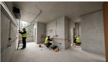
MEPS LINE INSTALLATION
